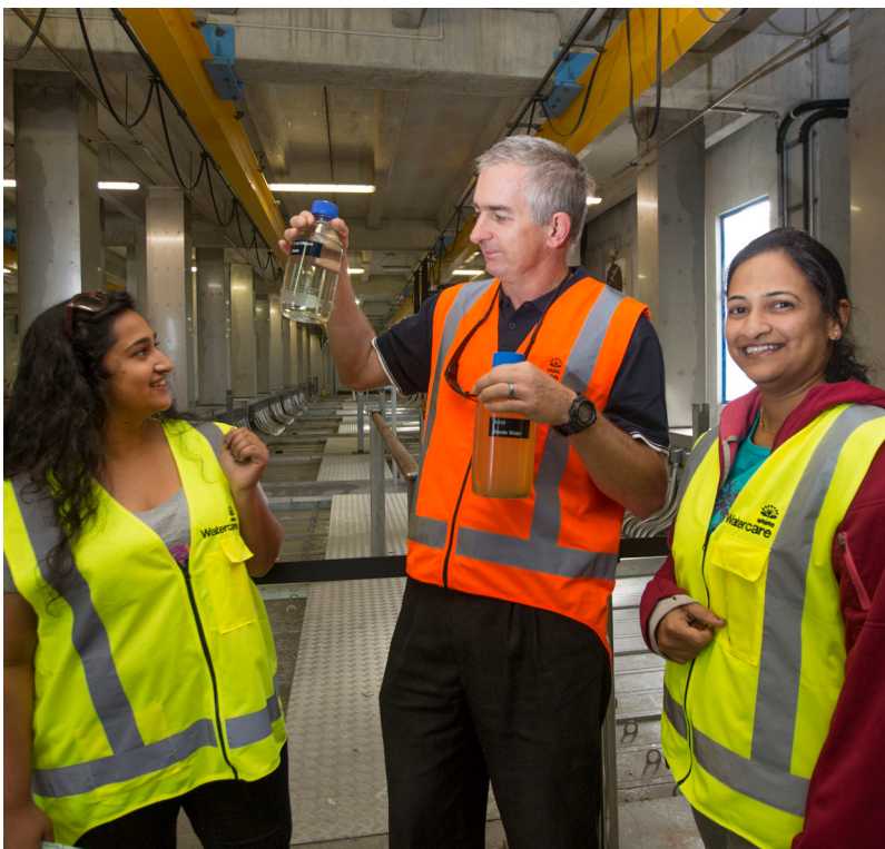
Maintenance controller Tim Burborough shows Parita (left) and Nita Dharmadhikari samples of raw wastewater as it enters the treatment plant, and the treated wastewater that leaves the plant 12 hours later.
